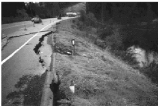
Road Section Before Repair
