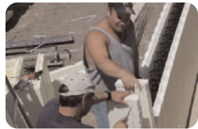
3 Cutting fillers: first 2 rows set the Advantage block pattern for the entire project
