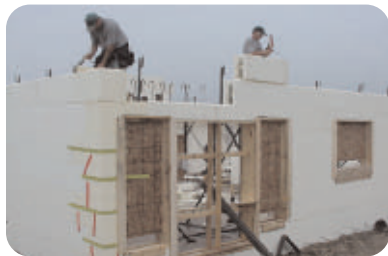
7 Place steel over doors and windows: stirrups may be required; brace door and window bucks
