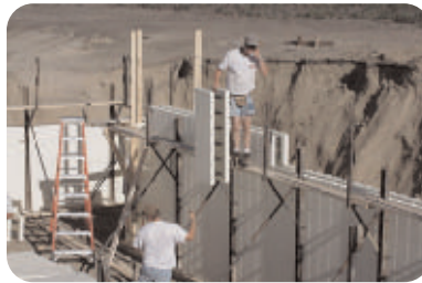
5 Work platform in place: continue setting block; follow the set pattern established in rows 1 and 2
