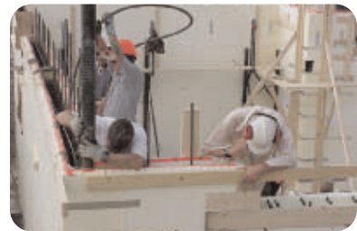
9 Placing concrete: make sure mix design is appropriate for job; follow proper placing techniques
