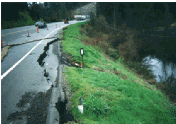
Figure 1 - Road Section Before Repair
